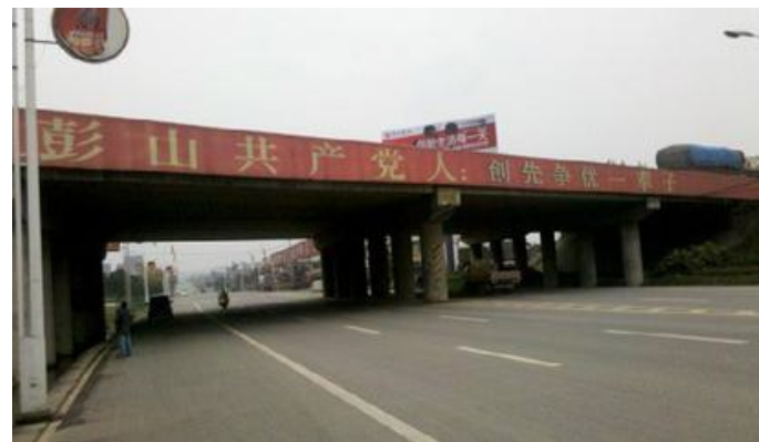
Before: The overpass was heavily affected by air pollution, causing visible dirt accumulation and surface discoloration over time.
